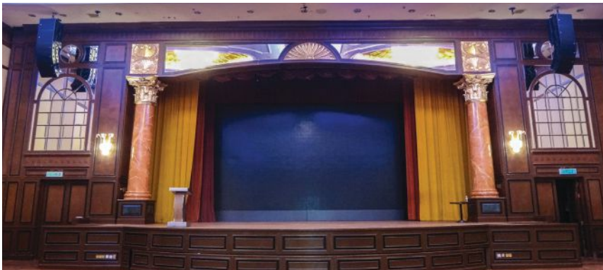
Renkus-Heinz CFX-series arrays flanking the stage in ballroom 2 at the Grand Lagoon Ballroom.
