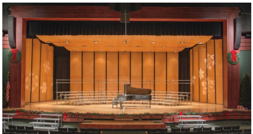
Discreet arrays made up of NEXO GEO M6 modules at left and right in the Swayne Auditorium.
